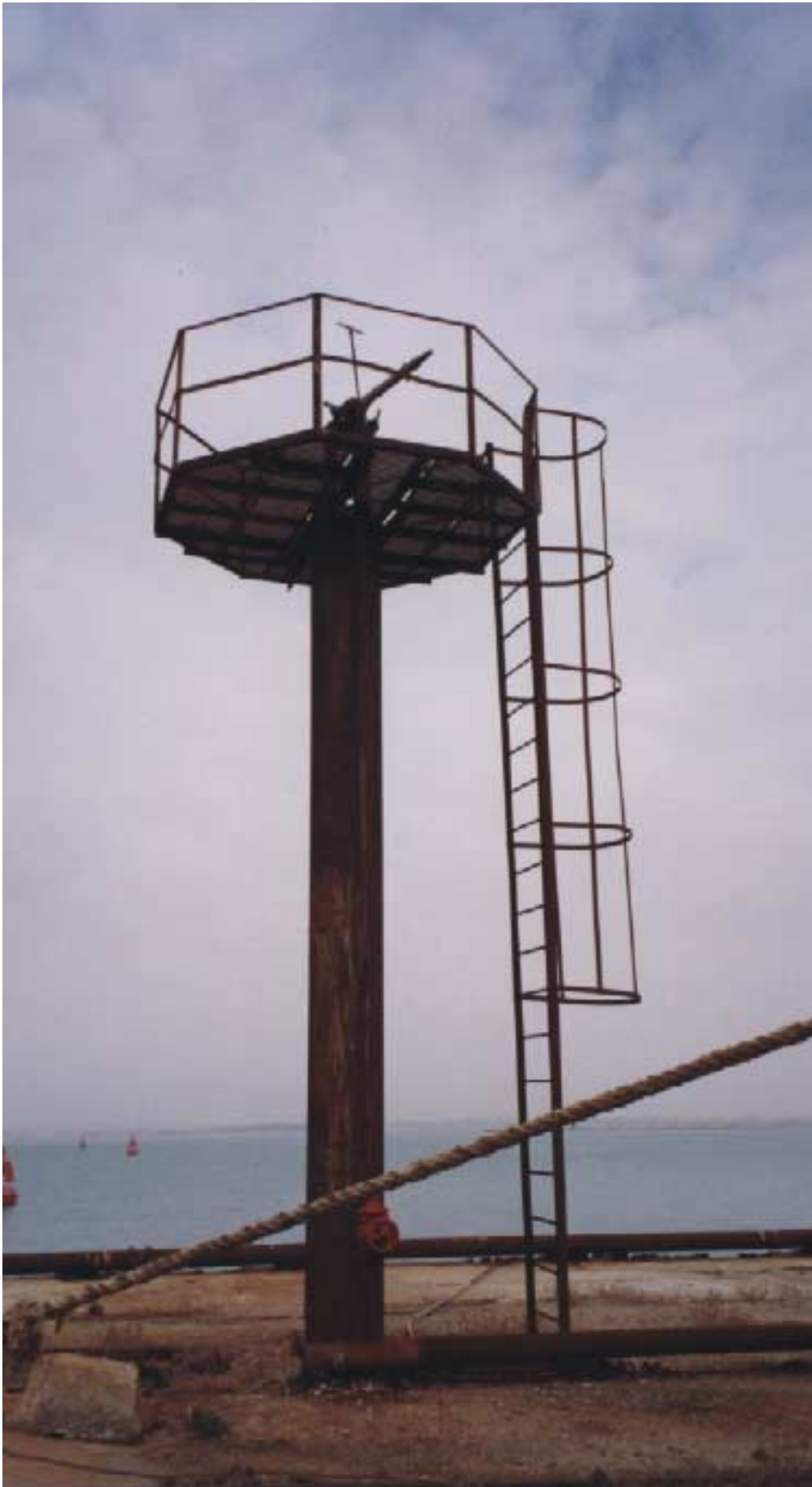
5. Fire-fighting tower between berths n°4 and n°5
